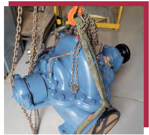
One of four High Service Pumps that maintain our water pressure and water supply located at the Filtration Plant.
