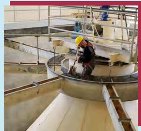
Regular cleaning and parts replacement each year.
